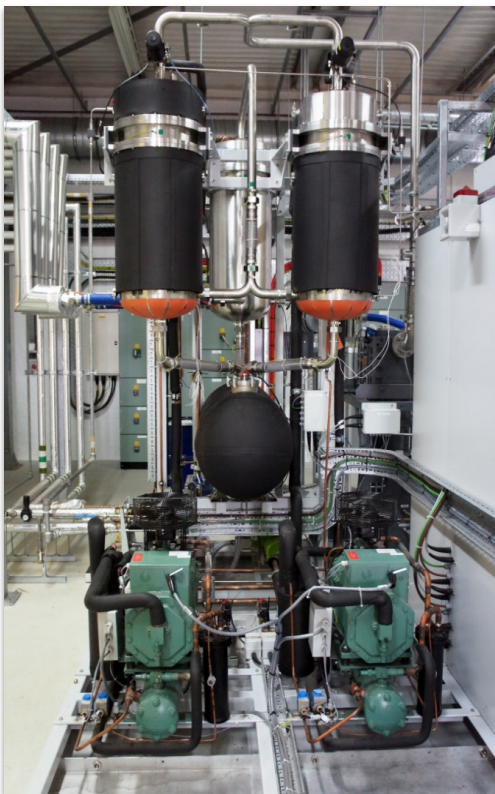
AVDS VACUUM CONDITIONING UNIT (VCU)
