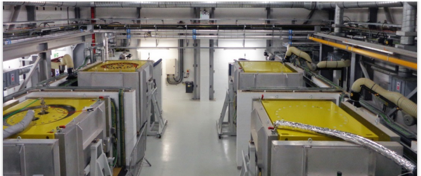
AVDS HEATING STATIONS FOR TYPE VI (CUBOIDAL) CONTAINER
