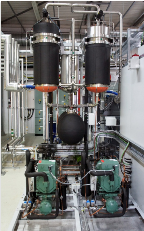
AVDS VACUUM CONDITIONING UNIT (VCU)
