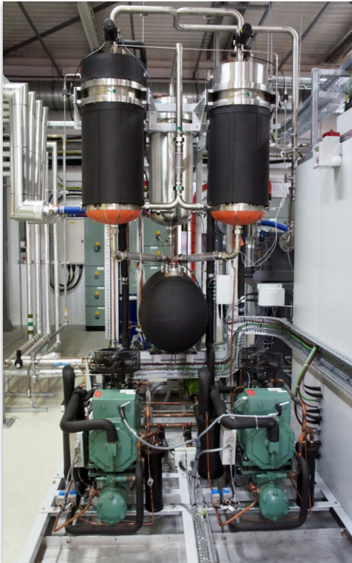
AVDS VACUUM CONDITIONING UNIT (VCU)
